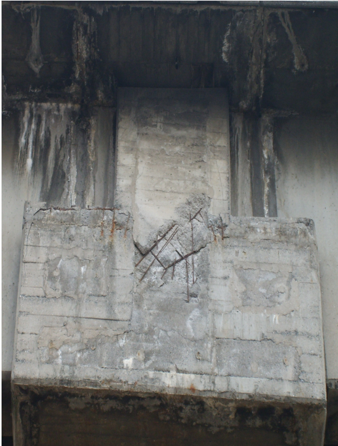
Figure 3.3. Corrosion at cross beam
