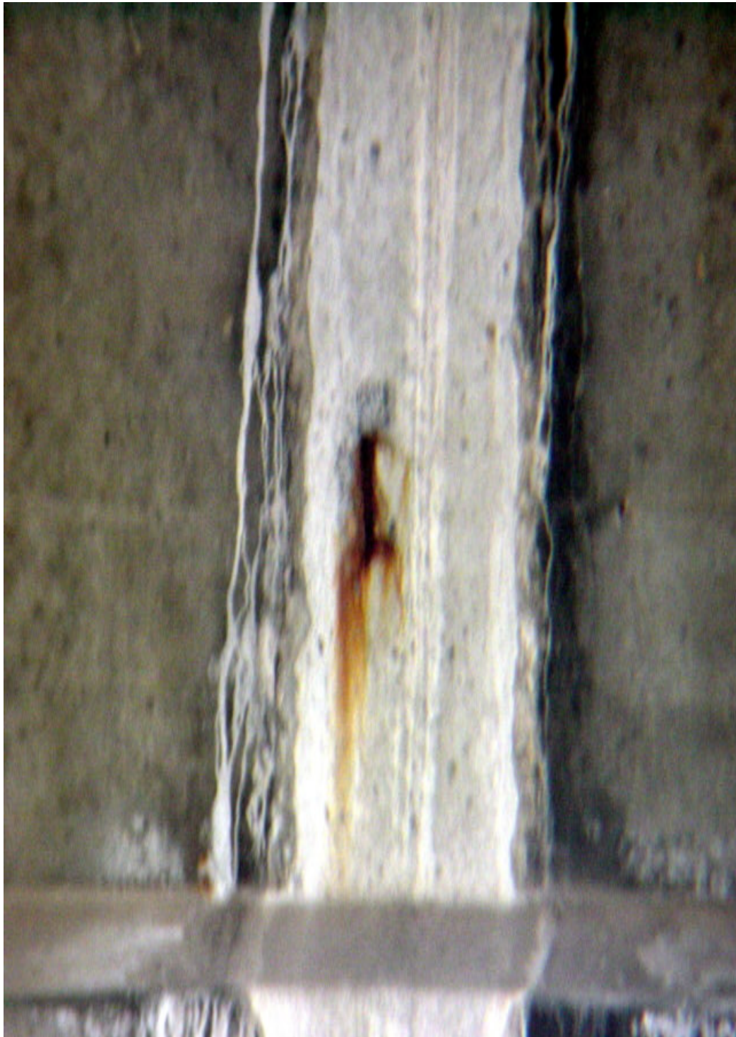
Figure 3.4. Corrosion at girder side
