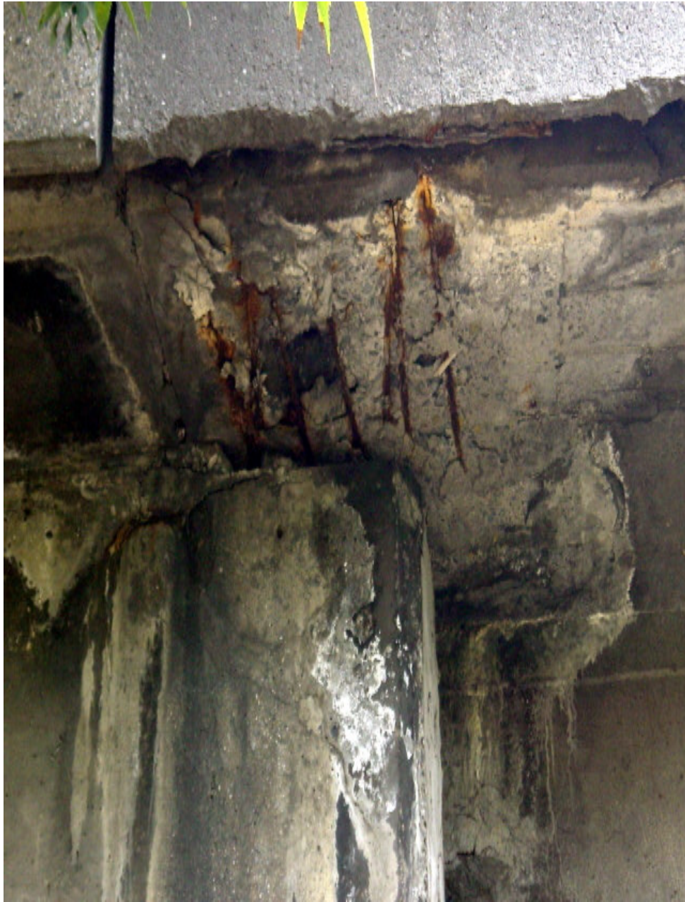
Figure 3.2. Corrosion at top of pier
