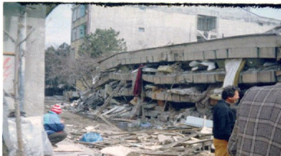
Figure 1.1. Collapse due to shear failure in columns (1992 Erzincan Earthquake)
