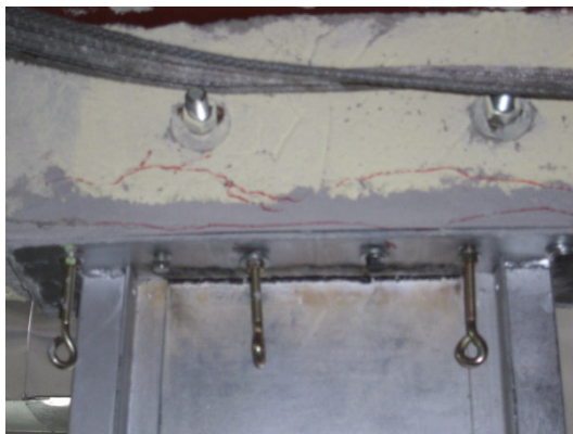
Figure 2.11. Shear failure occurred in the upper connection
