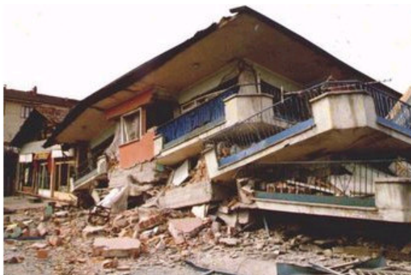
Figure 1.2. Collapse due to soft storey (1995 Dinar Earthquake)
