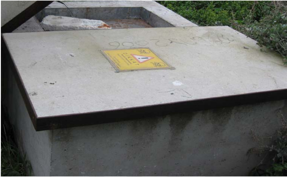
Figure B2. Photo of the PIREs Arrays stations housings on Sivriada and Yassiada Islands.
