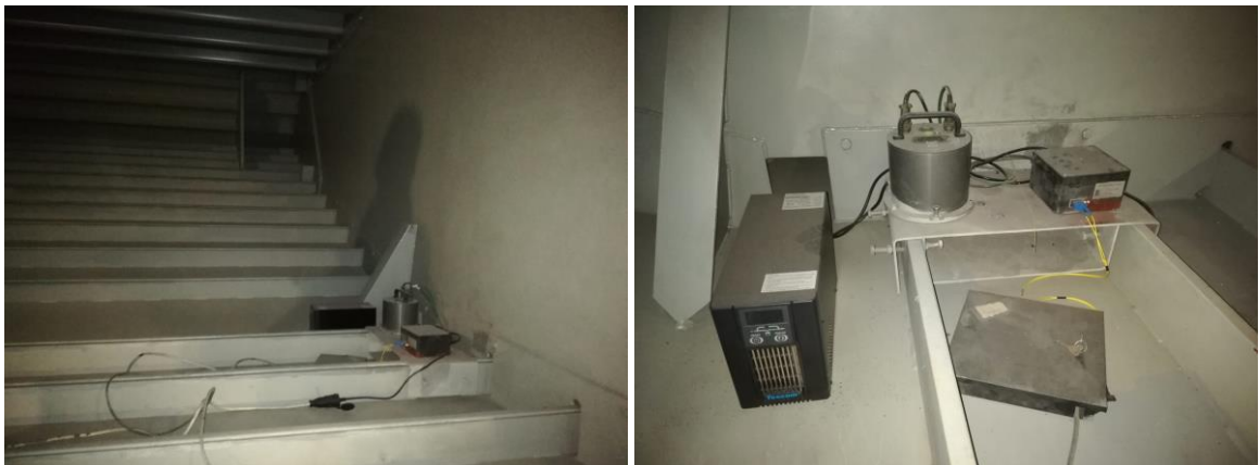
Figure 2.11. Permanent sensor inside the deck (number 10).
