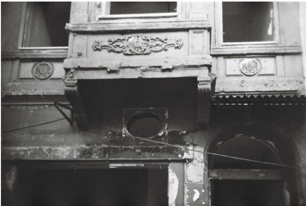
Photo 2: Detail on a house behind the fences, with doors and windows removed.
