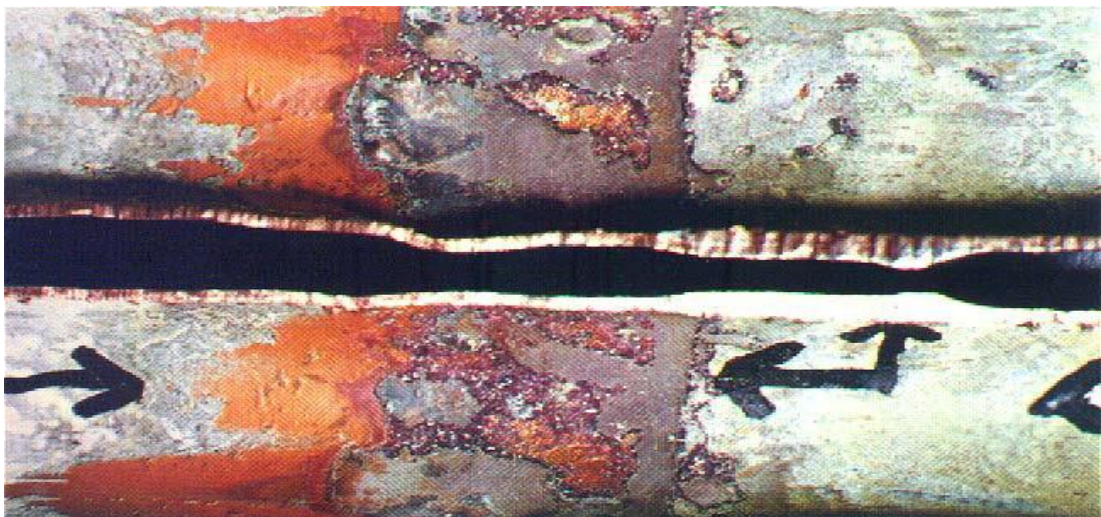
Figure 1.9 Erosion Corrosion in Solder Joints [13].
