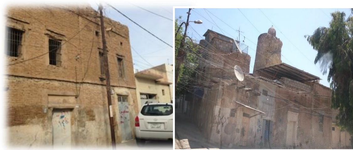
Figure 4.15 Irregularity of cables and electric system (Khasro et al. 2016).
