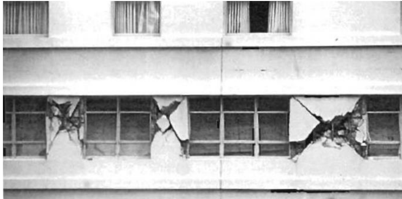
Figure 2.1. Failure of short column and shear wall, the Northridge earthquake.
