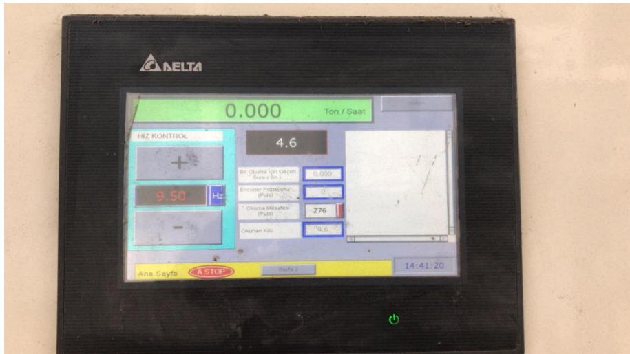
Figure 3.48 Weighing conveyor touch screen
