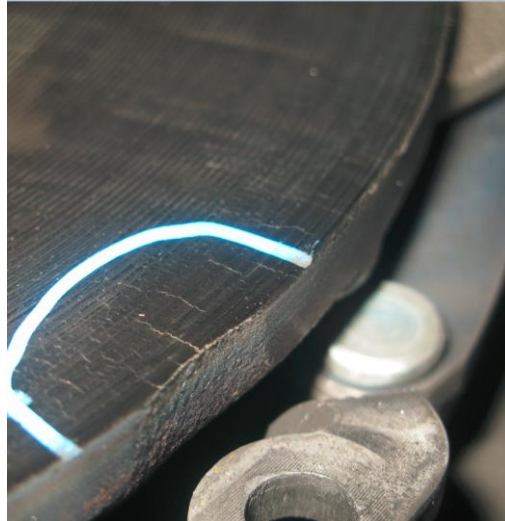
Figure 3.7. Test Part picture after thermal test with a crack on p.plate surface
