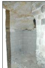
CONCRETE BRICK WALLS WERE CONSTRUCTED TO A CERTAIN LEVEL IN A WET SPACE
