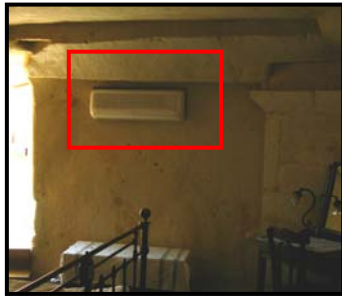
Figure 2.66 Air condition systems in rooms
