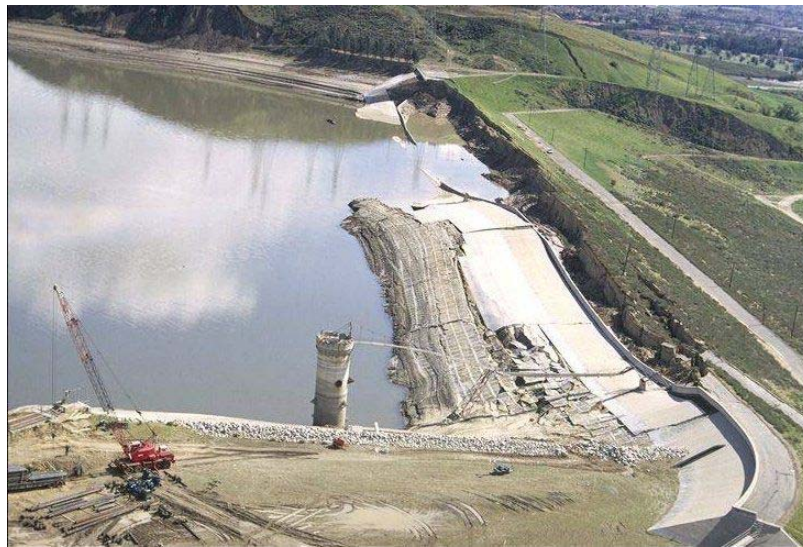
Figure 2.6: Lower San Fernando Dam Damage during San Fernando Earthquake, 1971
