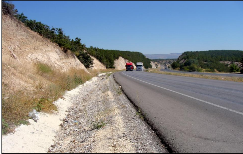
Figure 3.4. Example of a C slope with wide catchment and shoulder, a view looking toward Kurtboğazı Dam along D750 Highway.
