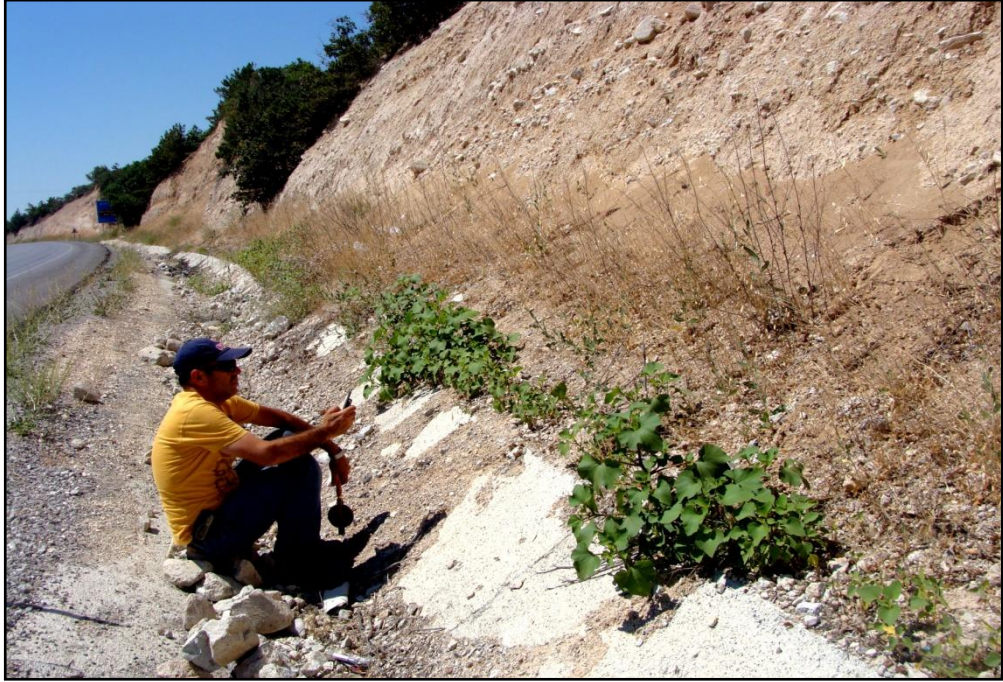
Figure 4.2. "C" rated slope near Kurtboğazi Dam, Ankara.
