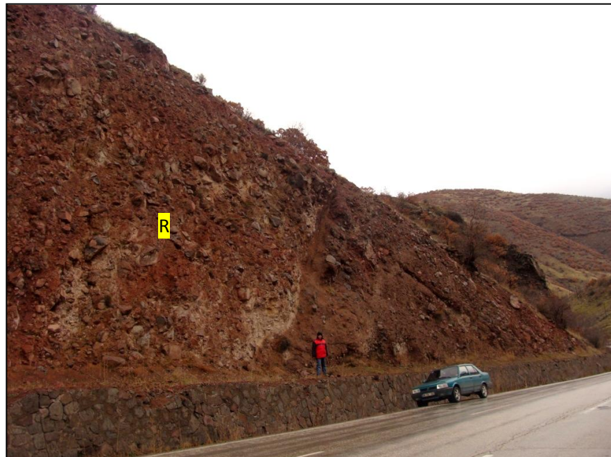
Figure 4.24. The figure showing the raveling mechanism in the “A9” rated slope Looking SE.
