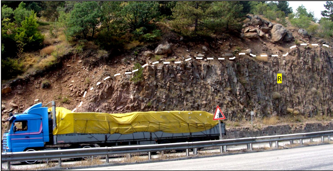
Figure 4.28. The figure showing the cut slope (“A12” rated slope”) which is opposite the A11 rated slope. Looking SW. The similar features are observed in this slope, too. The warning sign for rock fall is another indicator that these rock slopes may present hazard to the driving public. Note that the wall in front of the slope is demolished in some places.
