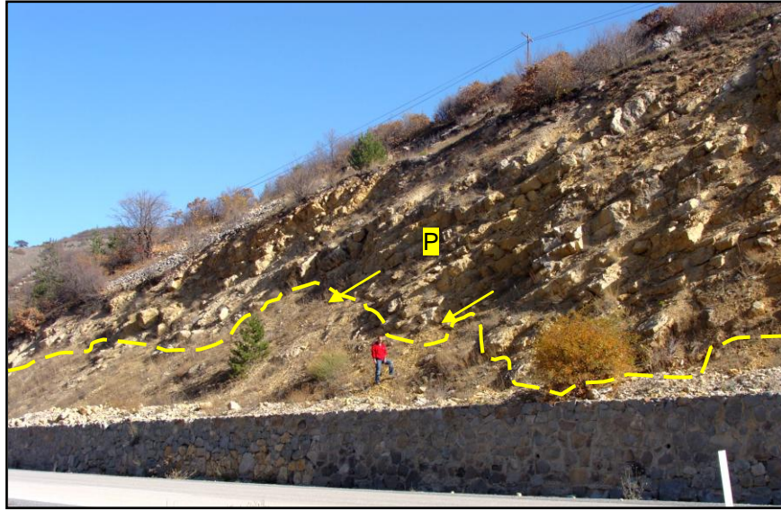
Figure 4.37. The limestone formation (Soğukçam formation, Aktaş region) which presents potential for planar slide in the direction of arrows. Looking NE.
