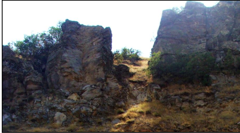
Figure 4.16. A close-up view to the top of the units of the rock cut. Looking NW. It can be seen that the rock blocks have potential to fail by wedge sliding. The gap which can be seen in the figure has been explained as the consequence of a failure occurred in the previous spring season by the local people.
