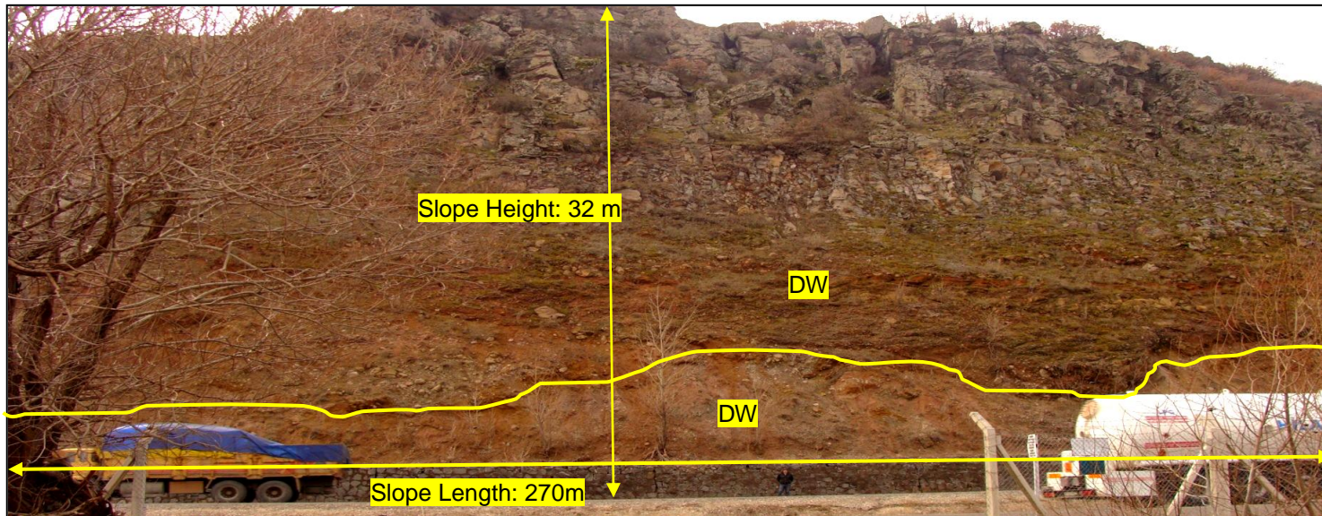
Figure 4.15. The view showing some of the features regarding site and roadway geometry and geologic characteristic of the “A3” rated slope. Looking NW. Note that this rock cut shows two lithologies with the lower unit eroding faster than the upper unit. Length of the rock cut captured in this figure is assumed to be the total length of the cut. An overhang is created along the boundary shown with the yellow line. Note that the boundary continues along the total length. Progression of the differential erosion may lead to loss of support of the more resistant unit above the rock cut.
