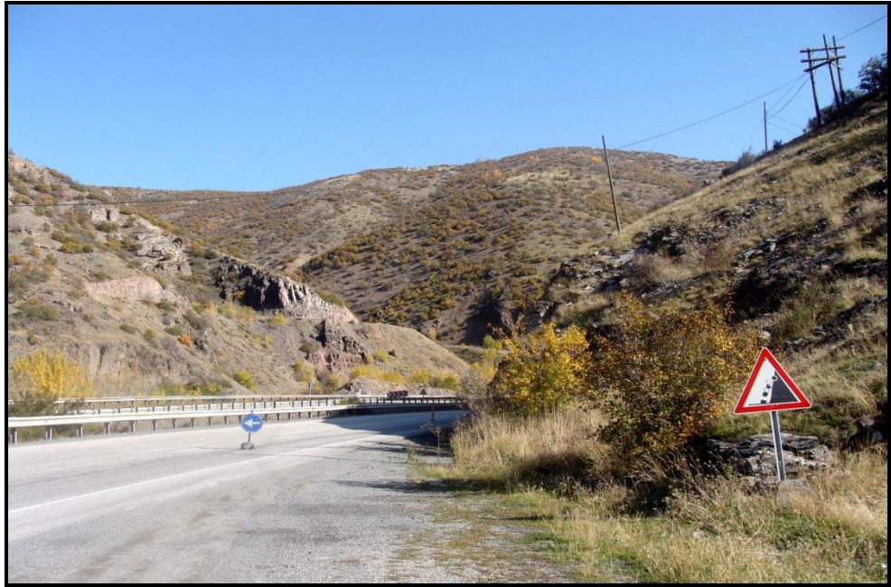
Figure 4.6a. The warning sign showing that the area is susceptible to rock fall events.
