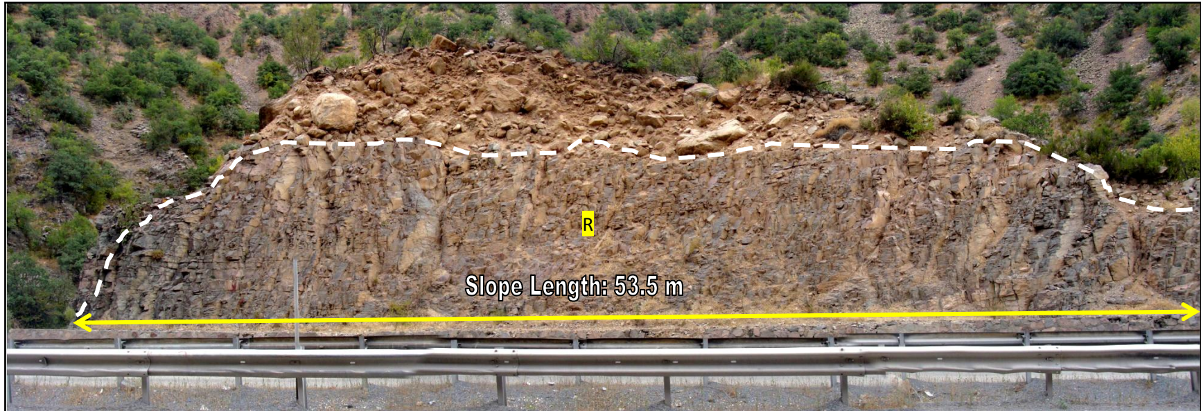
Figure 4.27. The figure shows the features of the rock face of the “A11” rated slope. Looking NE. It can be seen that the rock face under the dashed line is prone to raveling. The rock blocks at the crown part of the slope are prone to reach the roadway following heavy rainfall. The ditch is so narrow that it is hard to catch the rock blocks that may fall from the crown part.
