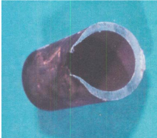
Figure 2.9 Fly ash erosion thinning and failure (EPRI Report, 2004) [4]
