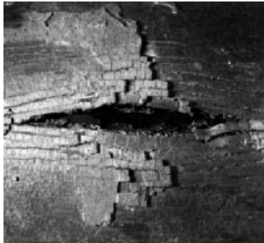
Figure 2.6 Long-term overheating (Babcock & Wilcox Company) [13]
