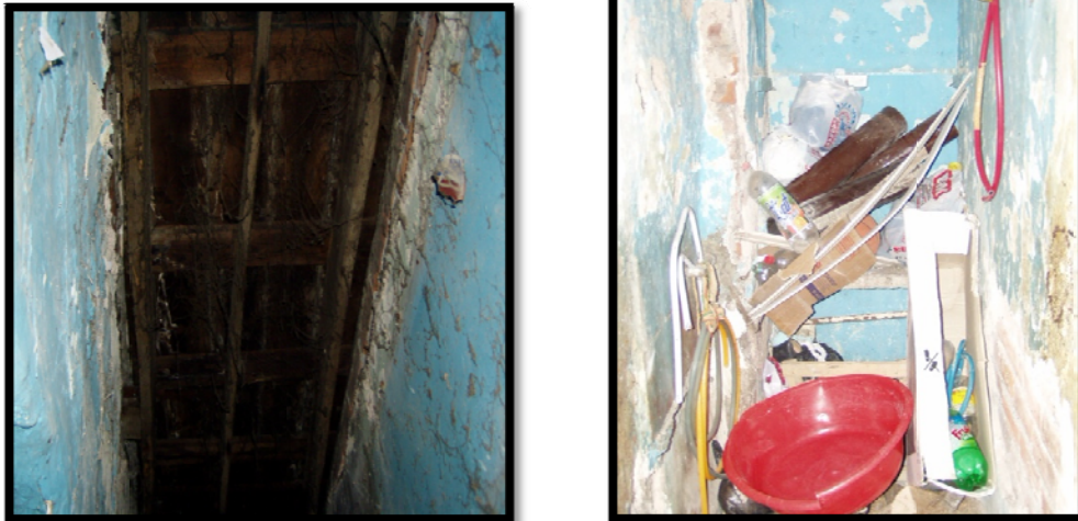
Figure 5.15-16: Unhealthy, neglected conditions of the houses (source :personal archive, 2004)
