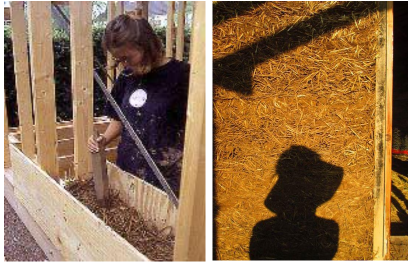
Figure 17: On the left, tamping process of straw LWL is seen (Gaia Architects 2003). On the right, climbing formwork and texture of straw LWL wall surface is shown.
