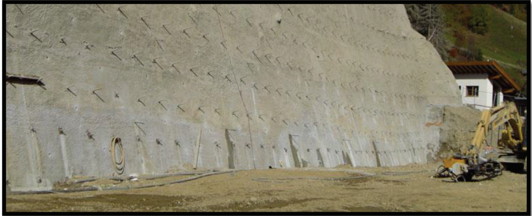
Figure 2.5 Horizontal drainage system installed on the retaining wall to reduce pore water pressure (Ischebeck Titan, 2016).
