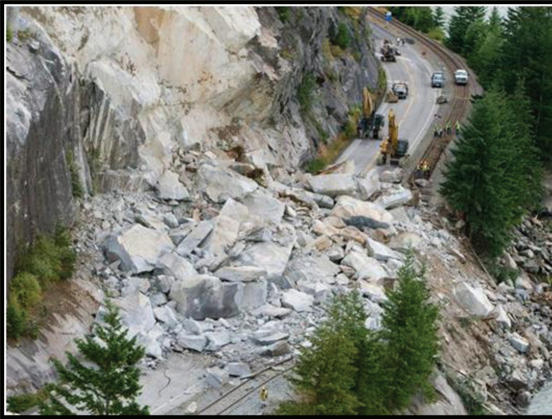
Figure 2.1 A rockfall event blocked the highway Sea to Sky joining Vancouver to the ski resort Whistler (Volkwein et al., 2011).
