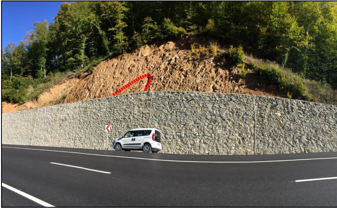
Figure 34. General view of the cut slope at Stop 4 (Failure zone indicated with red dashed line)
