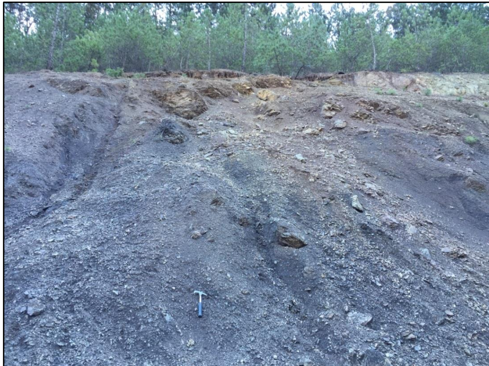
Figure 24. Failed zone of the cut slope at Stop 1
