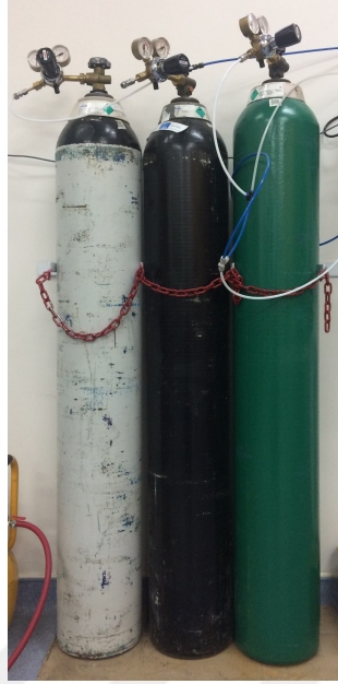
Figure 3.22 Gas cylinders located at Clean Combustion Laboratory. Green one is nitrogen cylinder used in pyrolysis experiments.
