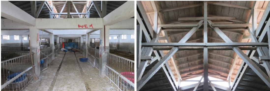
Figure 3.129. Interior view of the stable (on the left) and its timber roof structure (on the right)
