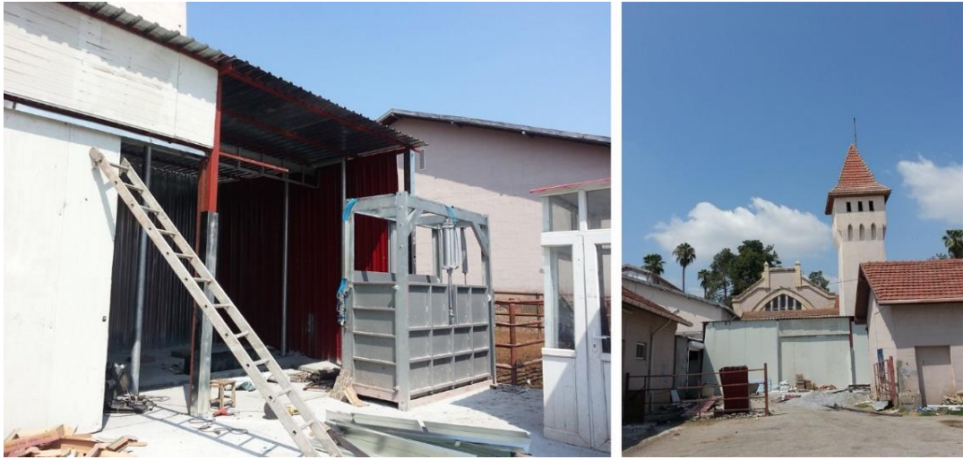
Figure 3.93. During the construction of the additional slaughter hall in August 2016 (Source: KUDEB archive)
