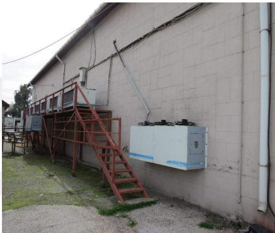
Figure 3.120. Air condition units mounted on the east façade of the building
