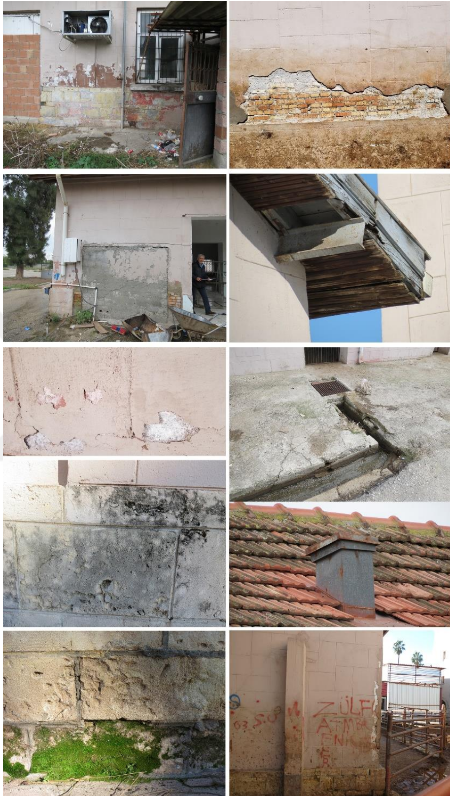
Figure 4.13. Most common problems detected inside the complex
