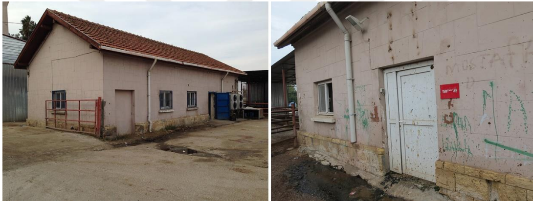
Figure 3.125. Exterior view (on left) deteriorations on the back façade of the building (on right)
