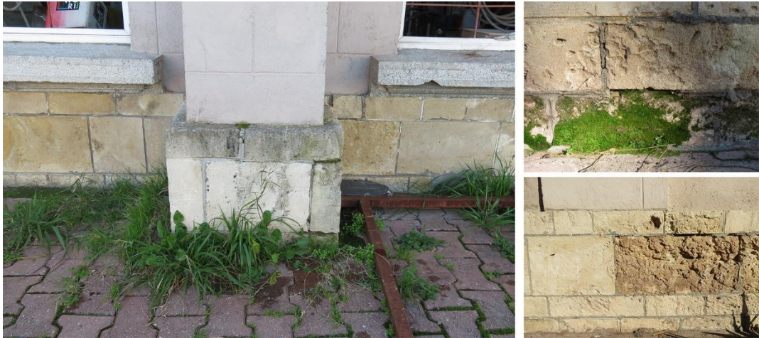
Figure 3.117. New material use for the renovation of stone (on the left) microbiological growth and material loss (on the right)
