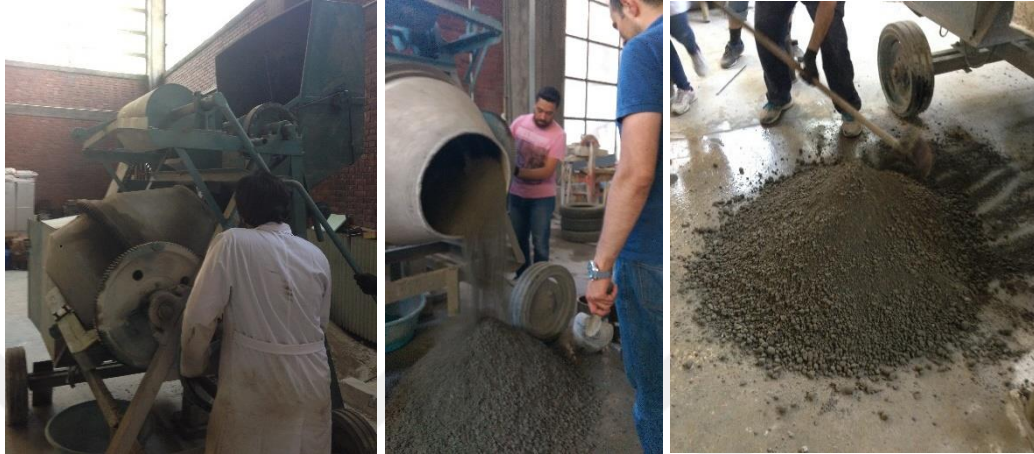
Figure 3.3. Mixing RCC mixture with rotary drum mixer and shovel on the ground
