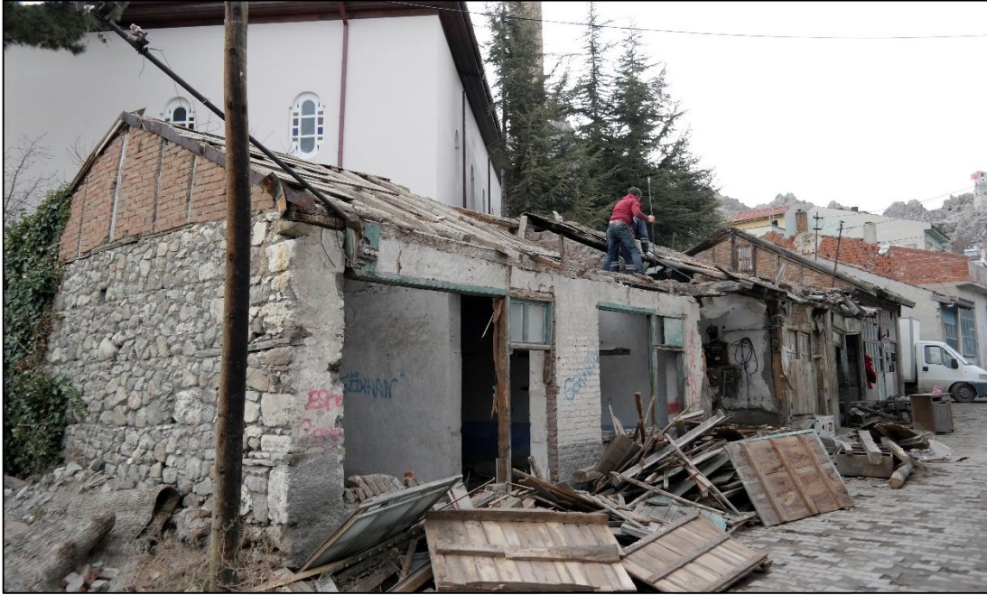
Figure 4-7. The Demolition of the Shops around Aziz Mahmud Hüdai Mosque (Author, December, 2017)
