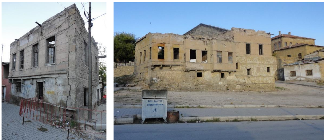
Figure 3.82. Abandoned buildings that has been destroyed (Personal Archive)
