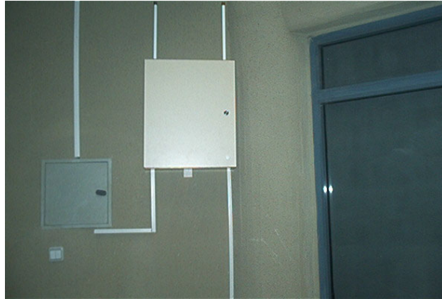
Figure 9 – Wood Enclosure for WLAN Equipment
