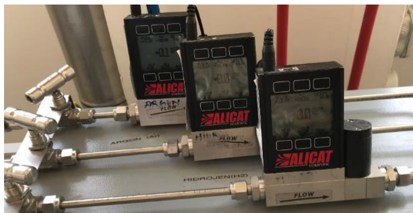
Figure 3-8 Carrier gases line (argon (Ar), hydrogen (H 2 ), nitrogen (N 2 )).
