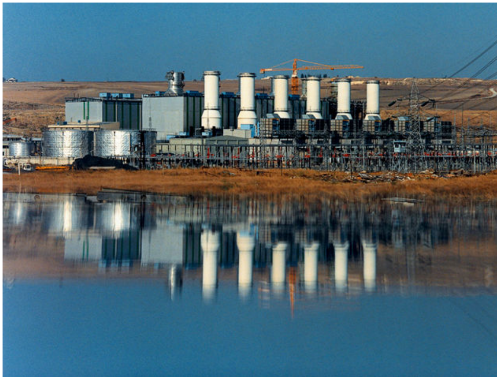
Figure 52: Ambarlı Combined Cycle Power Plant
