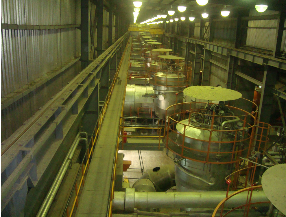
Figure 53: Ambarlı Siemens V94.2 Gas Turbines
