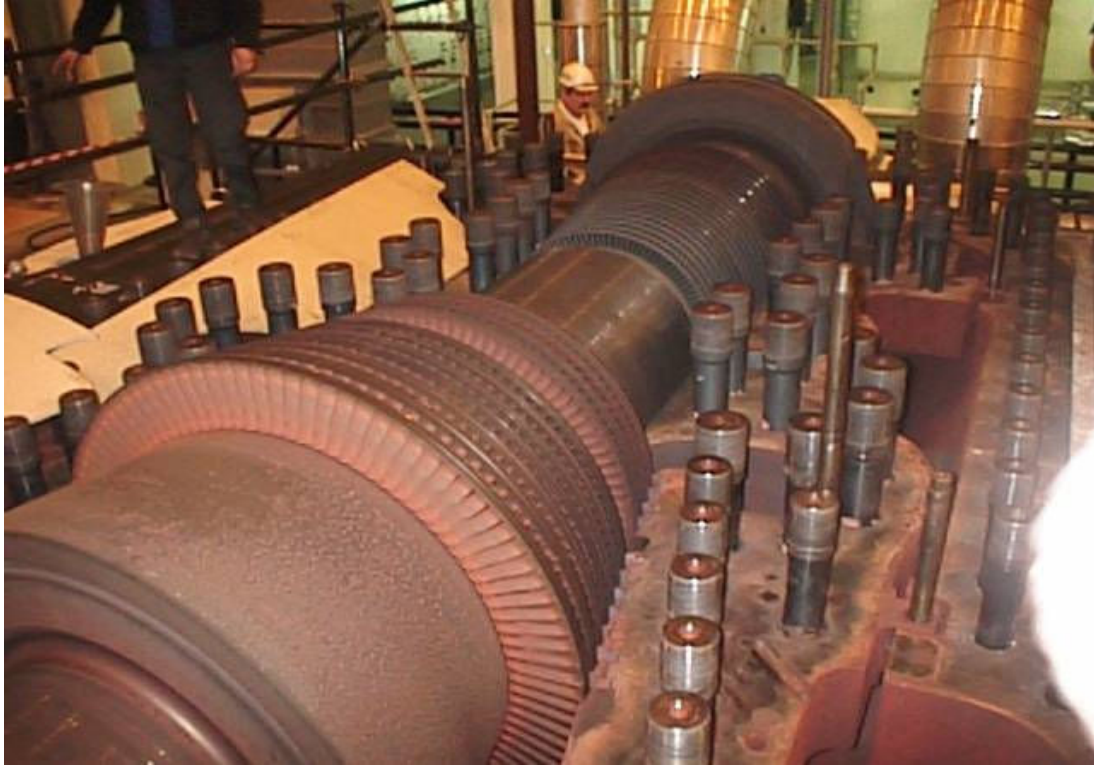
Figure 34: Degraded HP&IP Sections of a Steam Turbine
