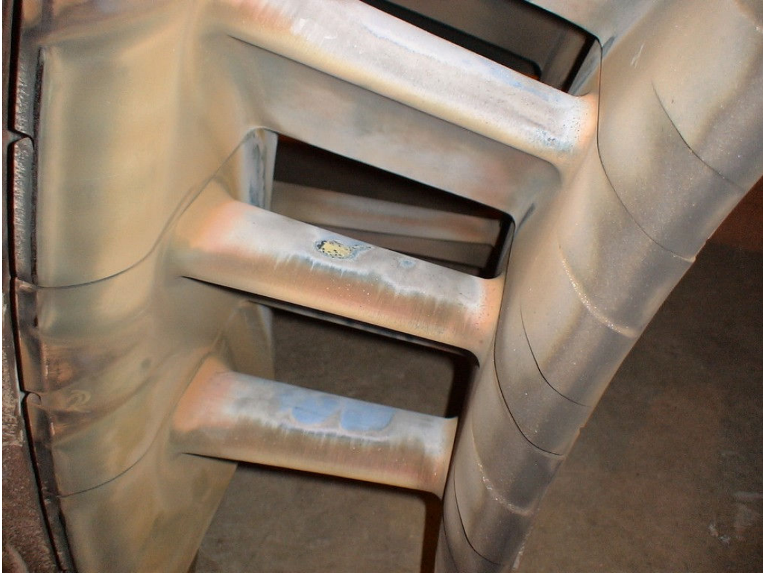
Figure 26: Eroded Coatings of the First Stage Nozzle
