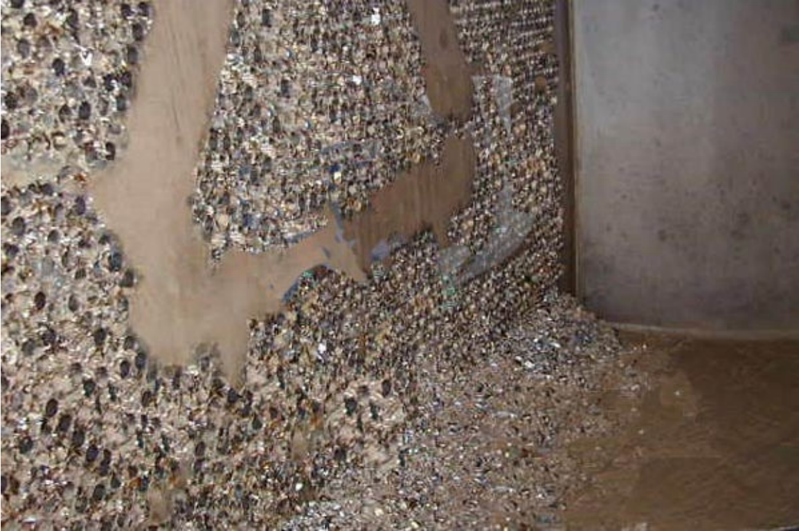
Figure 46: Clogged Condenser Tubes ( www.tubetech.com )
