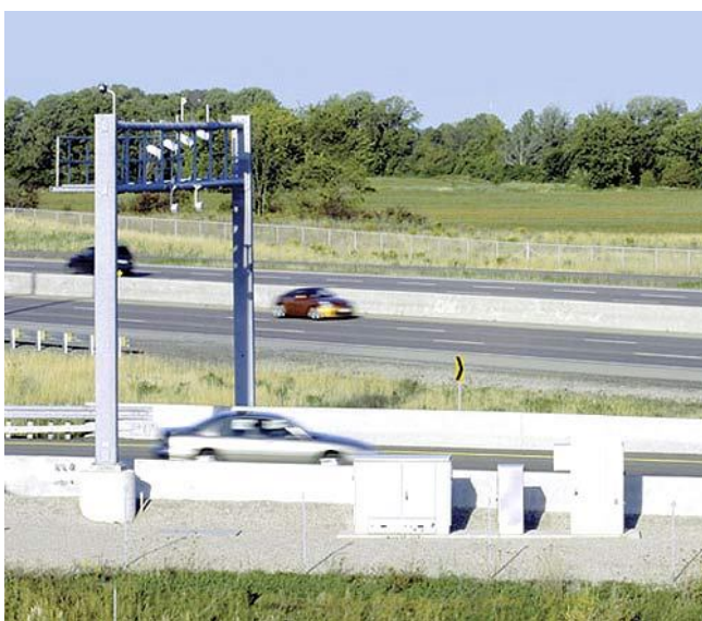
Picture 7.1 Control System at ETR-407 ("407 Express", 2009)
