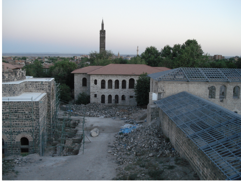
Figure 3: A view of the restoration works in progress in some of the İçkale buildings from one of the northern towers along the İçkale wall enclosure. On the left is the Church of Saint George, in the center one of the two Courthouses, on the right the Prison. On the background the basalt minaret of the Suleiman Mosque is visible.
