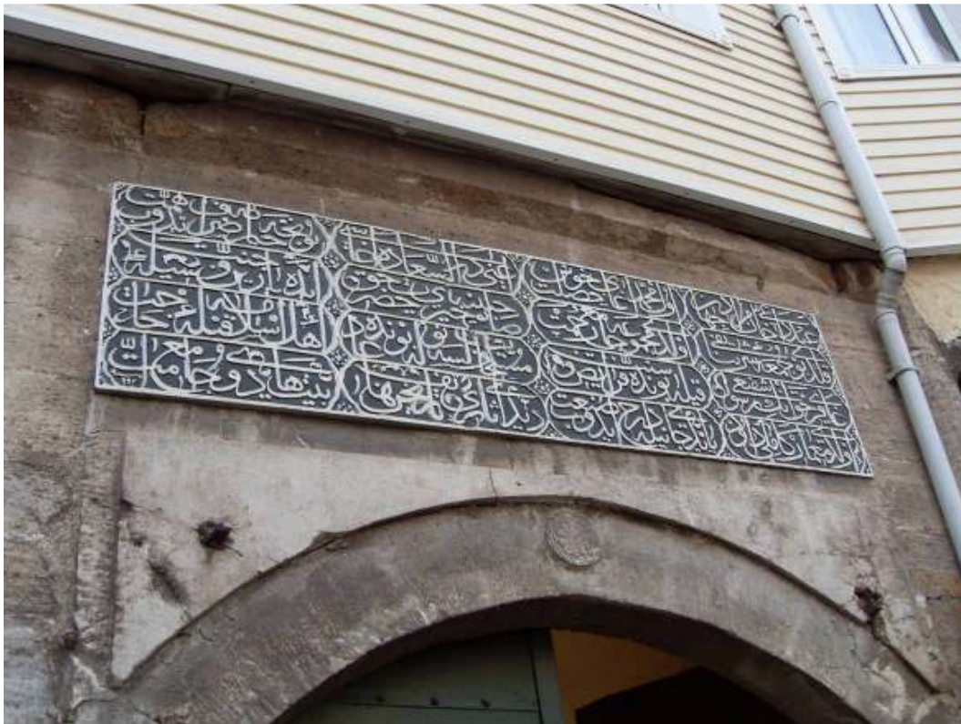
Fig. 40. The foundation inscription of the Habeshi Mehmed Agha Mosque above the entrance of the precinct
