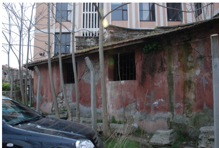
Fig. III.33 The ruined shed on the western niche of the church, 2010, (photo. by author).
