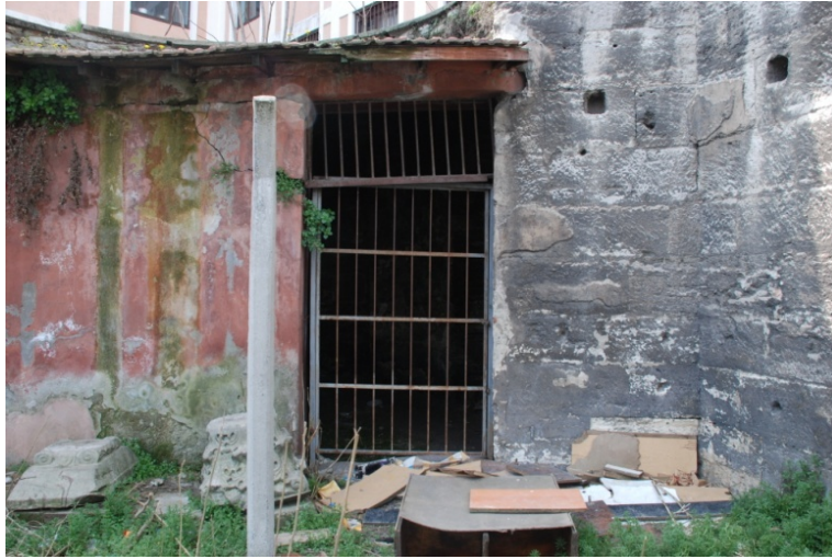
Fig. III.34 The ruined door of the shed, 2010 (photo. by author).
