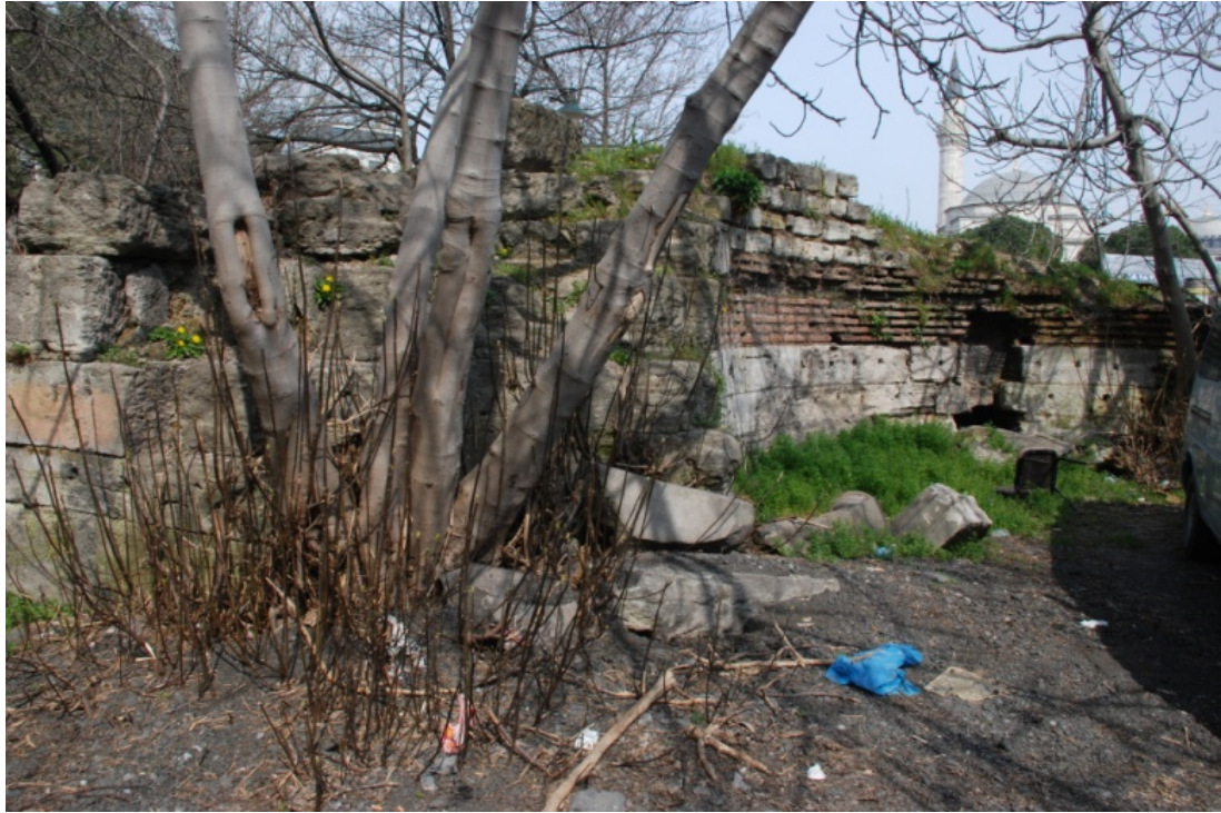
Fig. III.41 Roots of the plants cause structural damage, 2010, (photo. by author).
