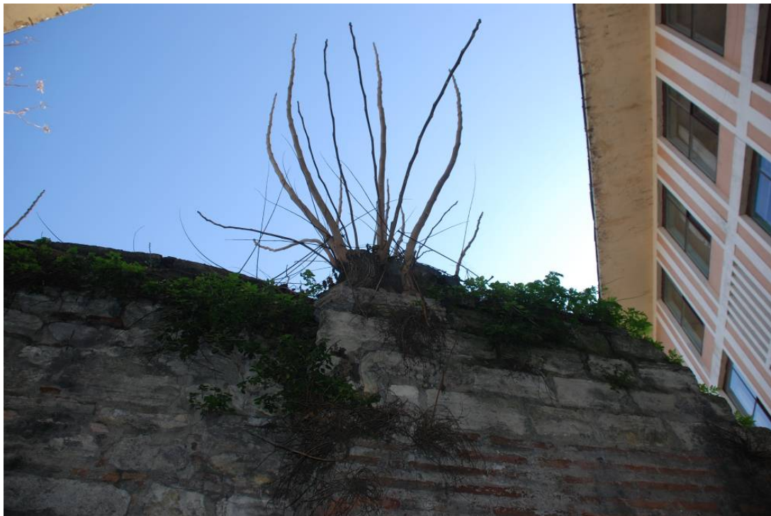
Fig. III.42 The damage of the uncontrolled plants, 2010, (photo. by author).
