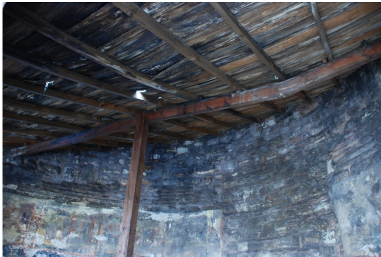
Fig. III.35 The dangerous roof of the shed, 2010, (photo. by author).
