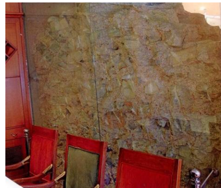
Fig 12 b: 6 th century wall after the conservation exhibited in situ in the Eresin Hotel
