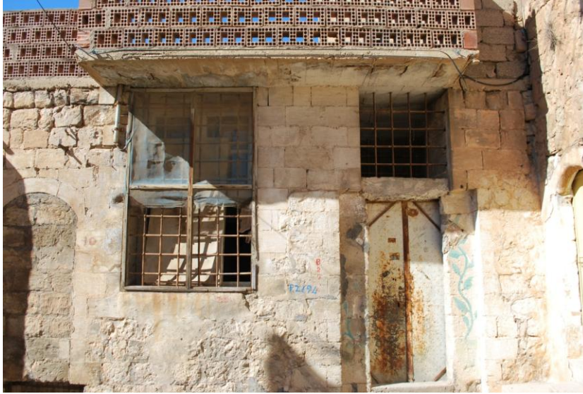
Figure 72 Unrestored building, Mardin. March 18, 2012. Photograph taken by author. JPEG file.
