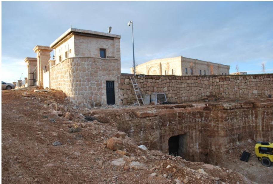
Figure 63 Construction of Visitor Center at Shiluh Winery, outside Midyat. March 17, 2012. Photograph taken by author. JPEG file.
