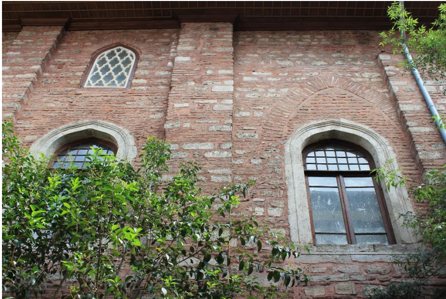
The trace of the original Gothic window on the southern façade of the Arap Camii. Photograph by the author, 29.07. 2018.
