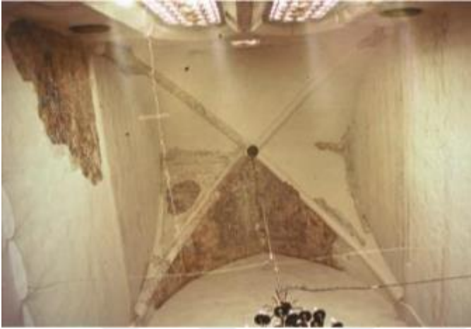
The ribbed vault of the apse, the Arap Camii, photograph taken after the 1999 earthquake. Akyürek, “The Frescoes of the Arap Camii,” 318.
