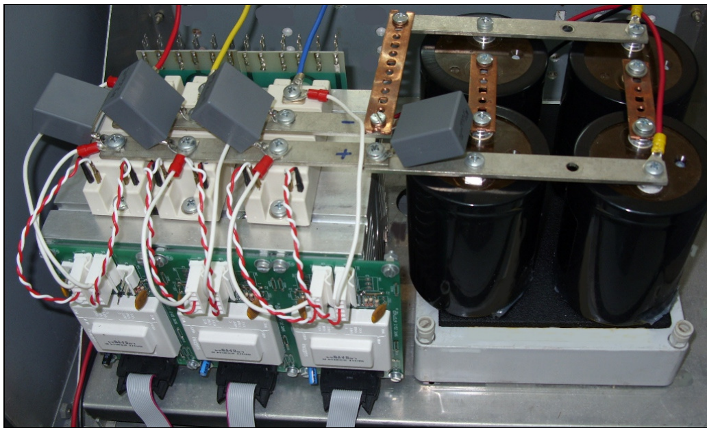
Figure 6.13. SAPF inverter with DC link capacitors
