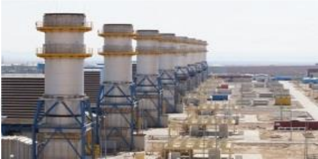
Figure 3.1: Duhok gas power station.
