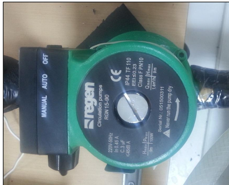
Figure (3.5): The hot water pump.
