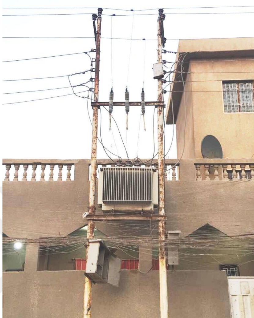
Figure 3.3: 250 kVA distribution transformer mounted on pole
