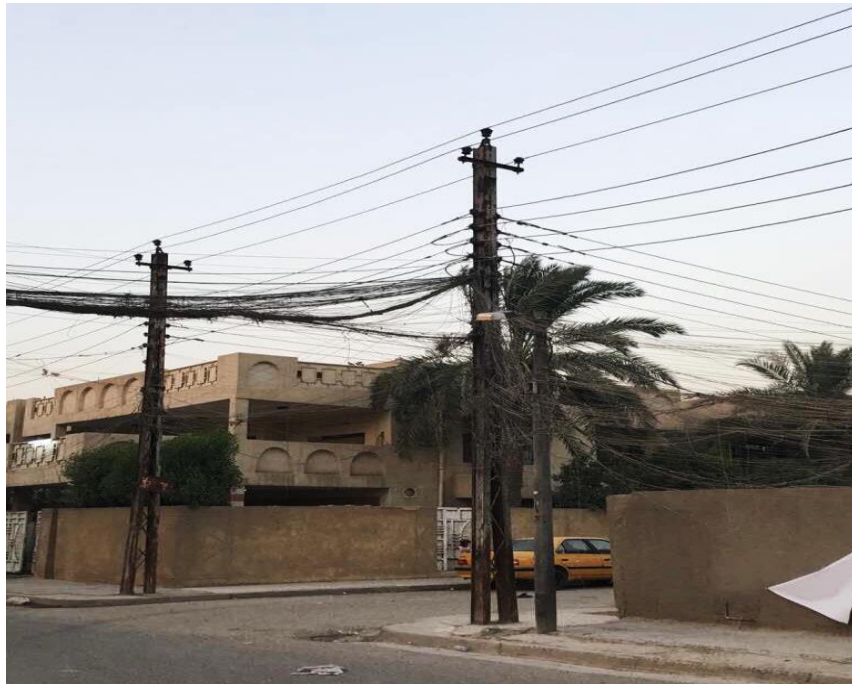
Figure 4.1: Baghdad City which the wires is naked and used in the air.
