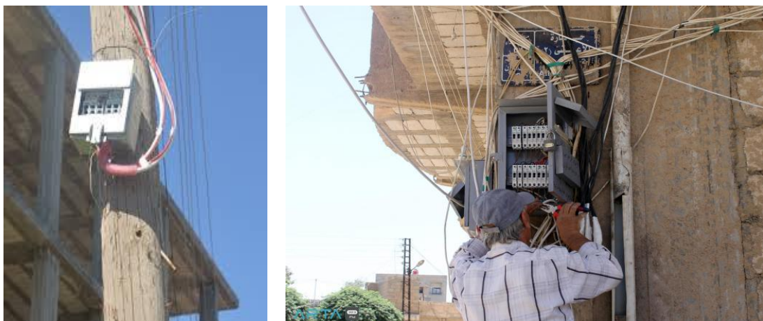
Figure 4.3: Connect limited circuit breaker (10 amperes) for each residence.
