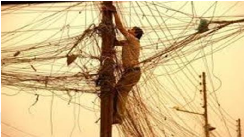
Figure 4.2: The illegal connection.
