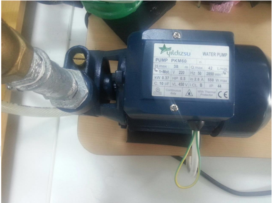
Figure 3.7: The cold fluid Pump.
