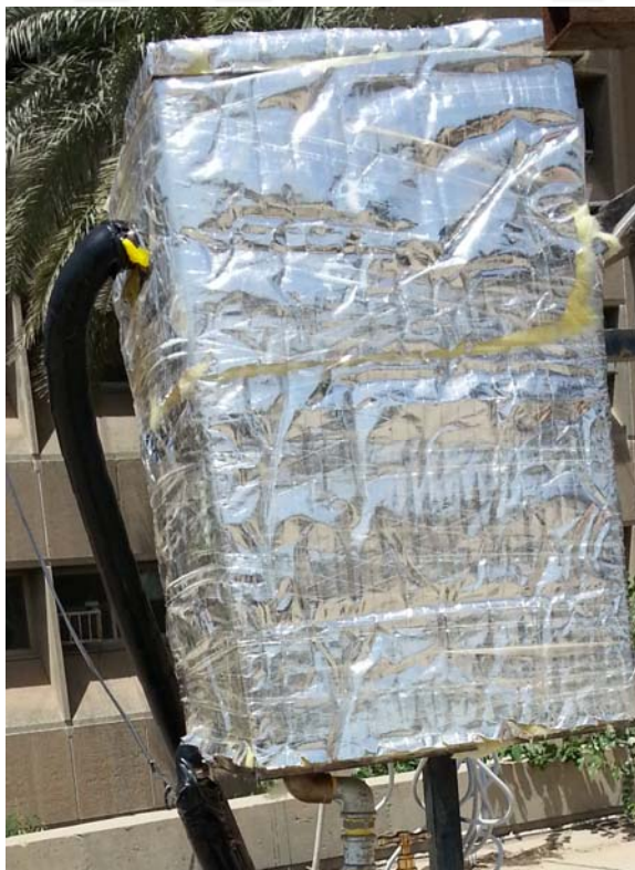
Figure 3.4: The insulated storage tank and the inlet and outlet pipes connected to the FPSC
