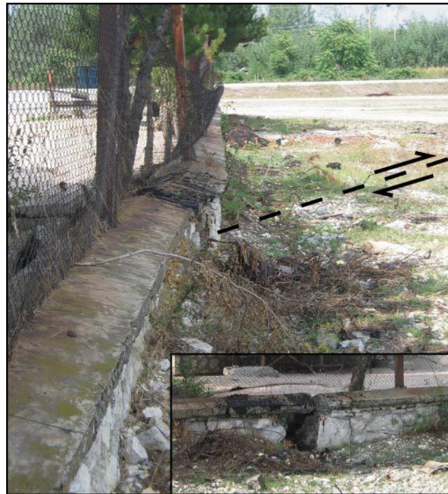
Figure 4.2: Photographs showing the warped and offset wall (~40 cm) due to fault-creep in the İsmetpaşa train station (September 2004, view towards the north). Note the extension of the wall due to the oblique cross cutting relationship between the wall and the fault in the inset photograph.
