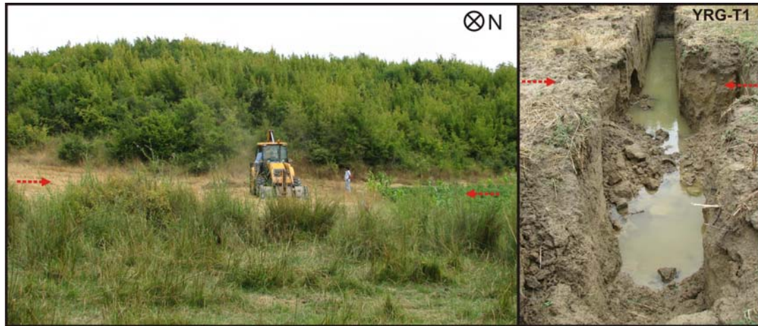
Figure 6.28 : View of the location of T1 at the eastern end of the basin. Red lines indicate the most-possible location of the fault zone. The presence of unconsolidated units and high ground-water level caused instability within the trench and walls collapsed when reached the fault zone.
