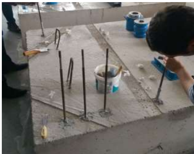
Figure 3.5 : Embedment of anchors.
