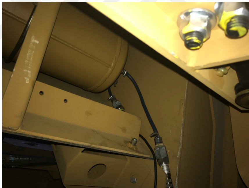
Figure 4.5 : Pressure sensors mounted on the front and rear tanks.
