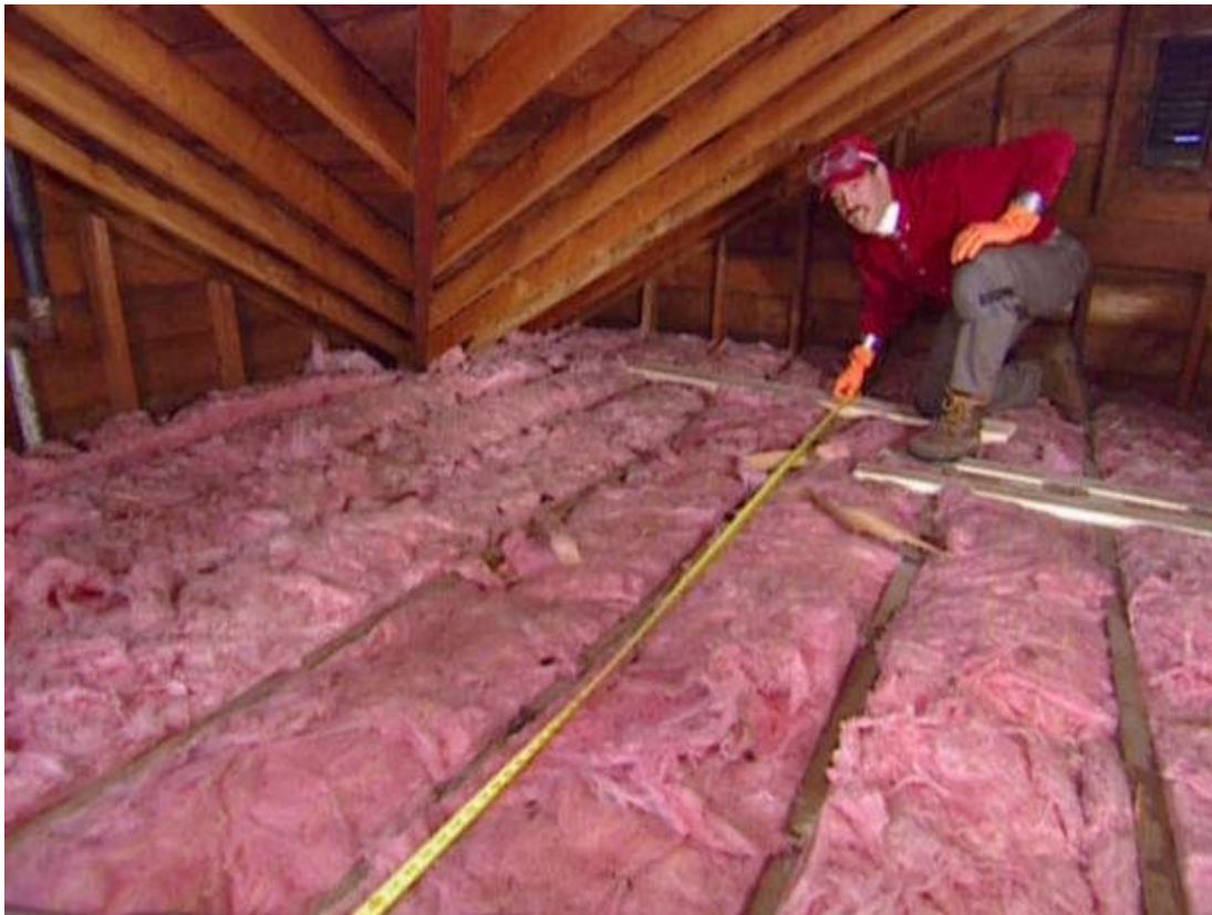
Figure 3.4 : Roof loft insulated with fiberglass.
