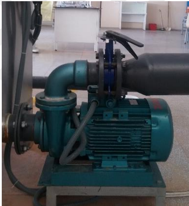
Figure 3.6 : Pump motor and butterfly valve
