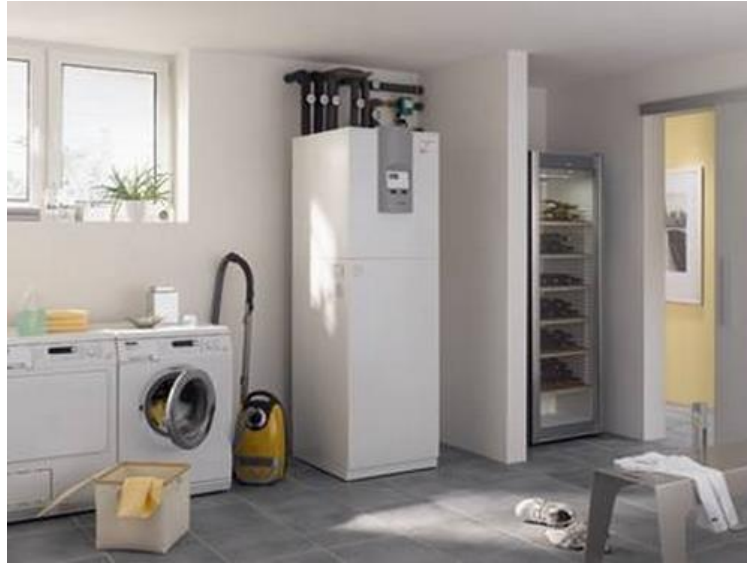
Figure 1.6: Small domestic ground source heat pump in home (EHPA, 2015).
