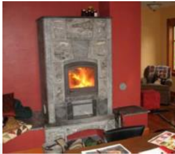
Figure 1.17: Photograph of Barkman family contraflow masonry heater, Pleasant Hill, Oregon (Hanley et al., 2005).
