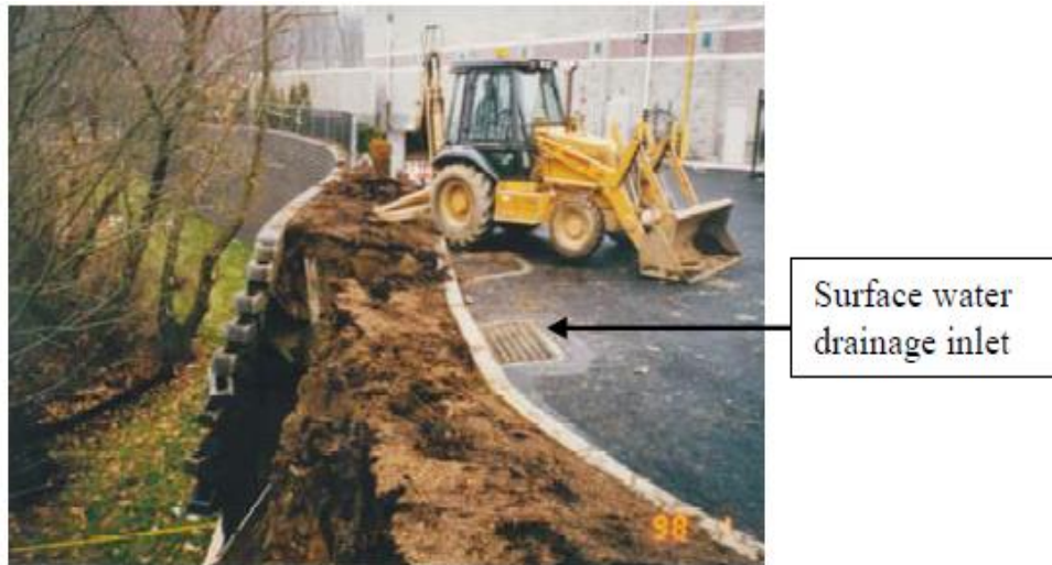
Figure 2.23 internal drainage failures (Koerner and Koerner, 2012)
