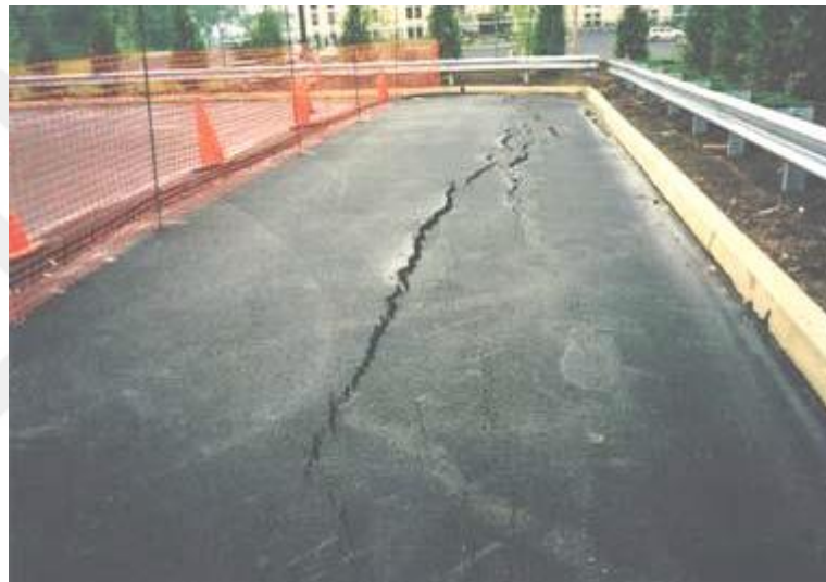
Figure 2.26 Tension cracks occurring exactly at the end of the wall reinforcement (Koerner and Koerner, 2012)
