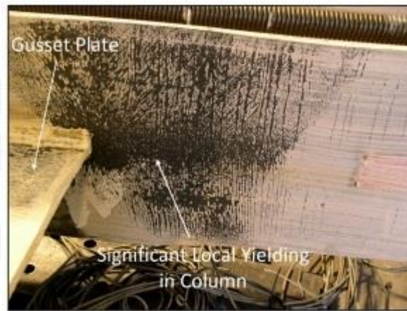
c) Local yielding in beam and column
