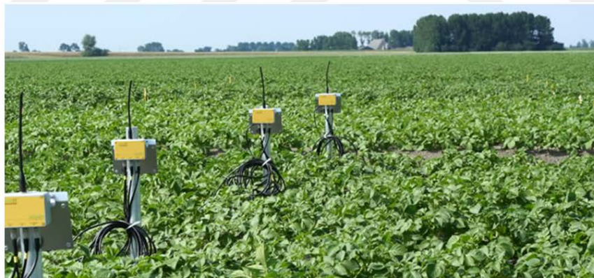
Figure 3.12: WSN agriculture monitoring by WaterSense Co. 2018, http://www.projectwatersense.nl/ [84].
